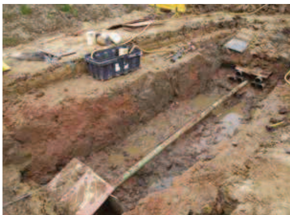
6. Excavate Joint Pit and Conduct Cable Pull (Post Duct Installation and Reinstatement)
